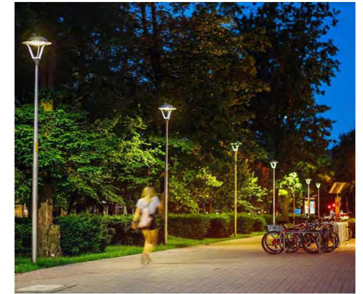
Column lighting to streets and courtyards.
