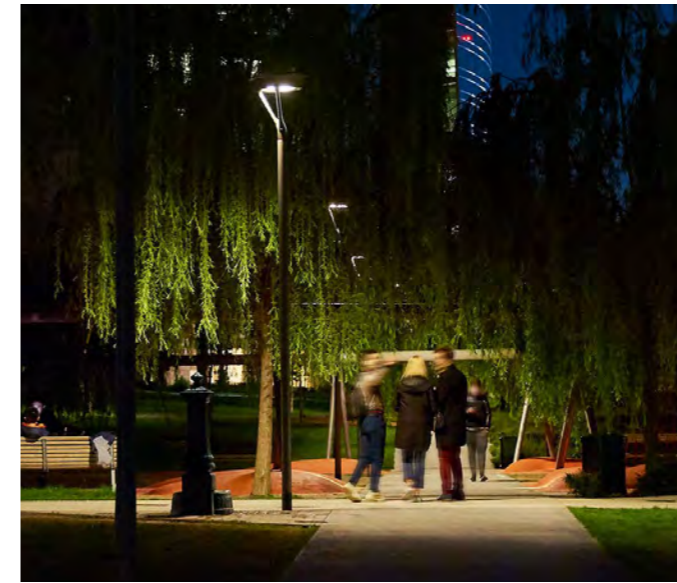
Column mounted luminaries along the primary movement areas in the Linear Park.
