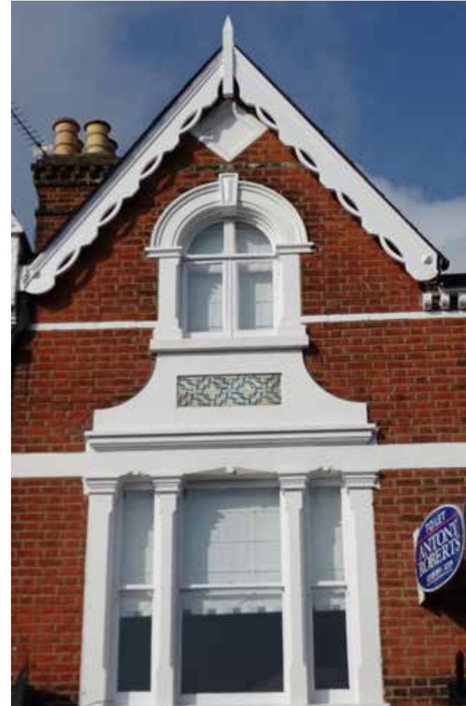
Timber casement window with white painted curved corning and tiled detailing below
