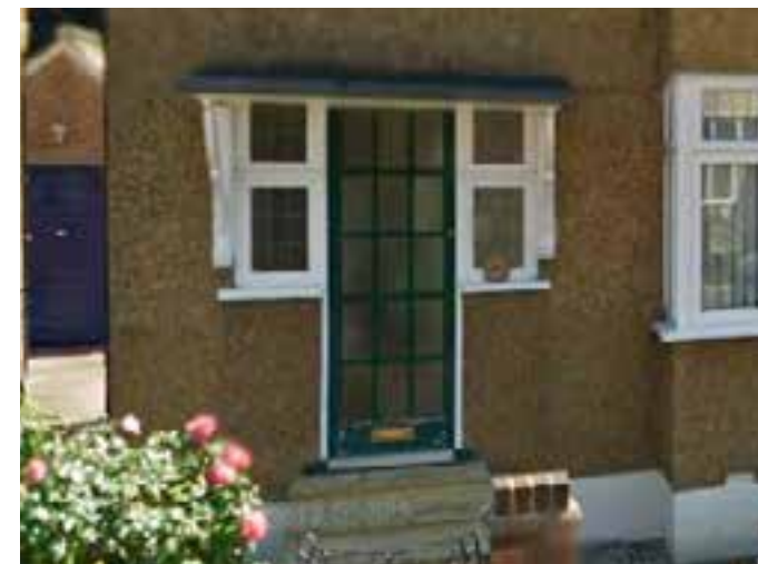
Flat or pitched canopies (on brackets). The example is a flat canopy over a door with side lights
