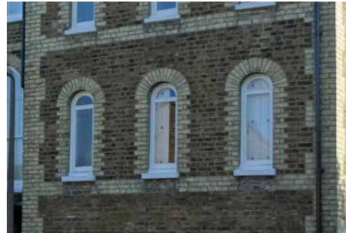
Round-headed Victorian Classical sash windows: to the left and arched upper sash has multiple panes; to the right, likely original sashes have been replaced with casements
