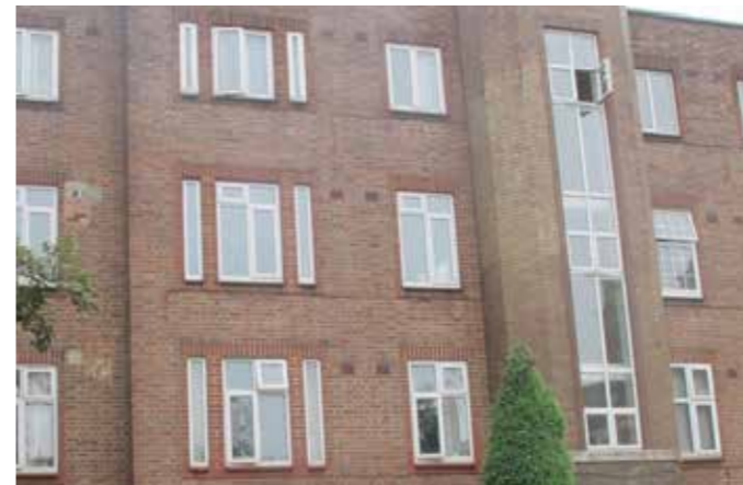
Art deco-influenced metal-framed windows with casement openings; many of those to the left and right have been replaced with uPVC window in differing styles, those at the highest level retaining the greatest sense of the original design
