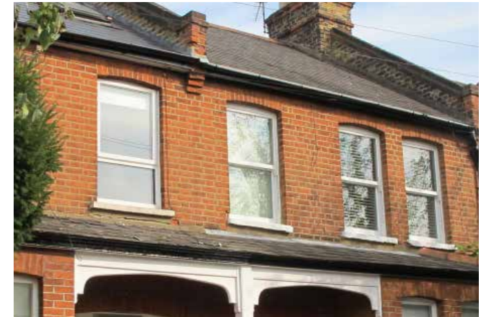
Later Victorian single-pane sash windows in reveals with a very shallow brick arch lintel
