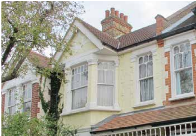
Late-Victorian hybrid sash windows in a canted bay with Classical-moulded reveals, the upper sash containing an arcade motif of shaped panes framed in fine timber girdles
