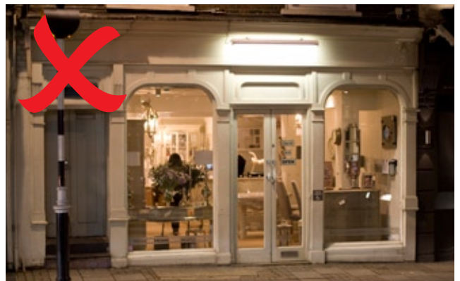
Fascia signage should state the name or trade of the premises and its street number
