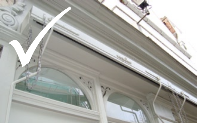
An original style awning and other decorative detailing has been retained and reused to good effect
