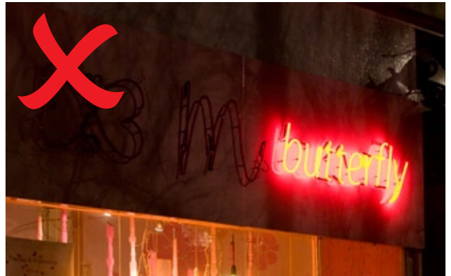
This is an example of where lighting has either not been switched on or not working
