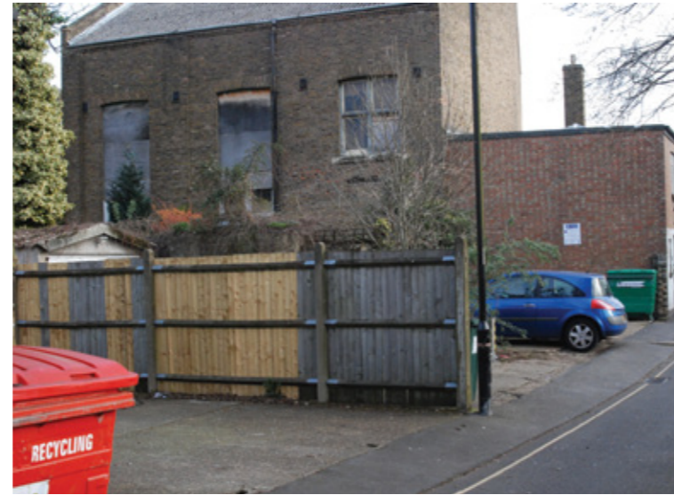
Queen's Hall, in need of restoration
