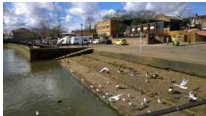
Need to improve stepped access to river and landing facilities
