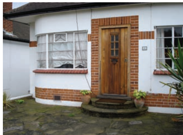
2. Original details – fenestration, brick bands, roof tiles. Inappropriate alterations: front garden paved over.
