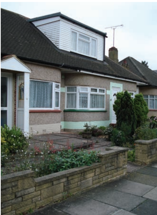
4. Original details – roof tiles. Inappropriate alterations – pebble dashing to elevations, brick bands painted over, box roof dormer, front garden paved over, porch, fenestration.
