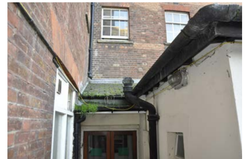
Figure 53: Blocked rainwater goods
