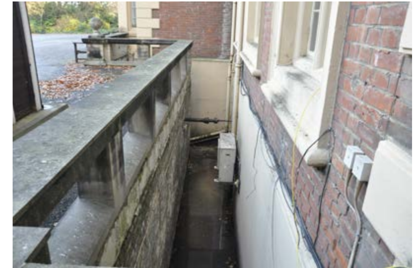
Figure 56: Blocked drainage network at northern lightwells
