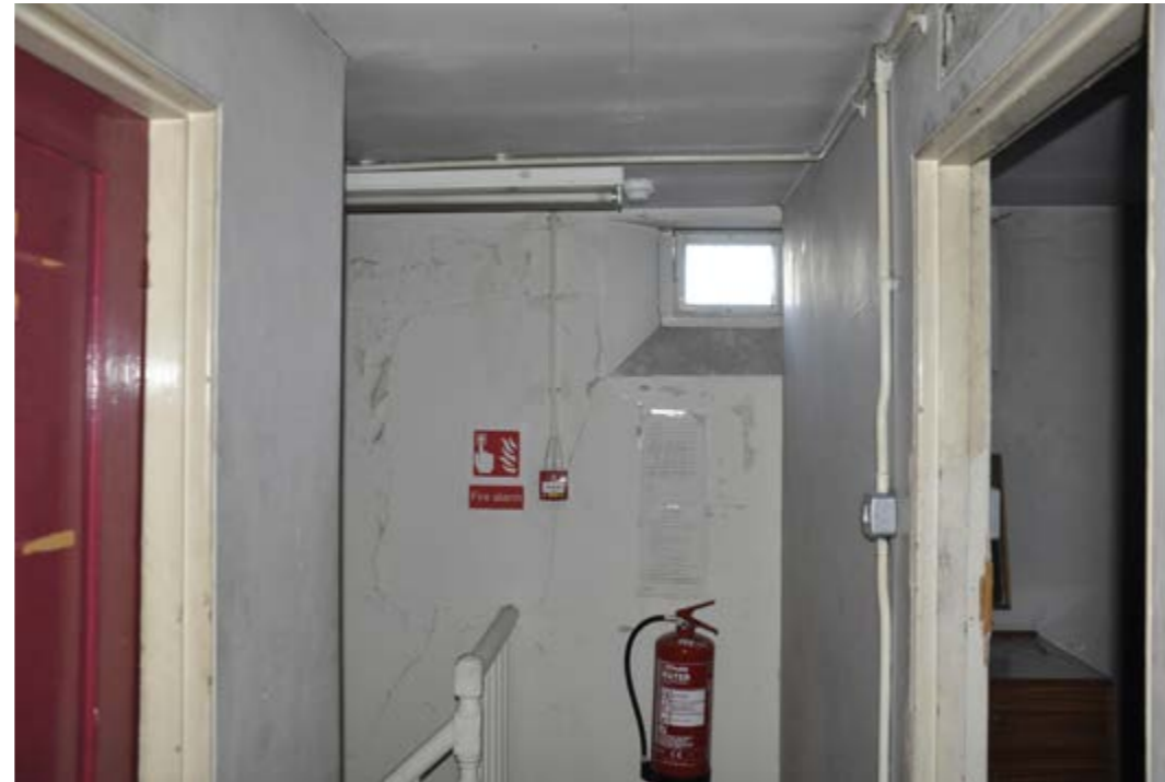
Figure 58: Signs of water ingress in the loft
