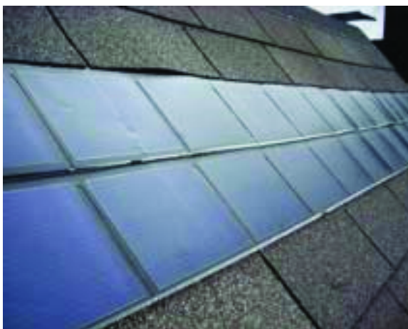
Image 35: Integrated solar panels
