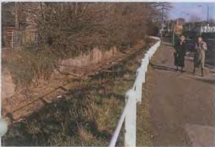
Fig.97 The ha-ha between Kew Road and the Old Deer Park has suffered from decay, damage and the straggling growth of scrub trees along its top
