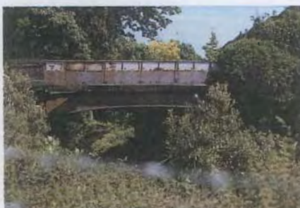
Fig.90 The railway bridge would benefit from maintenance
