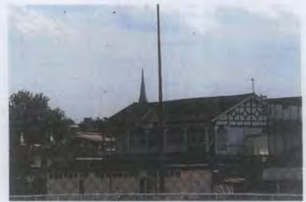
Fig.102 The northern front of the Grade II listed pavilion has been blocked off by a concrete extension
