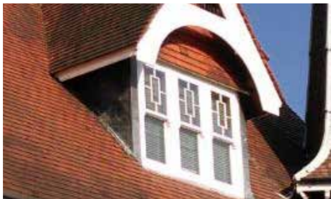
Sash window with attractive glasswork detailing and white painted barge board above
