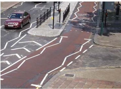
Red surfacing with wrong type of finish
