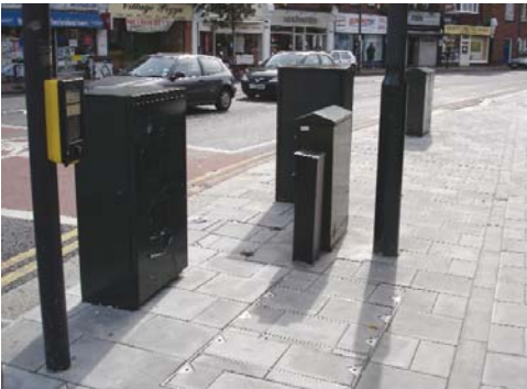
Poorly sited cabinets
