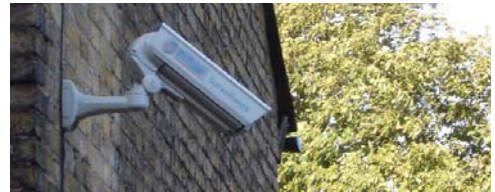
CCTV camera sited on building
