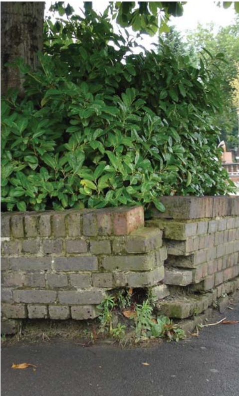
Raised planter problems
